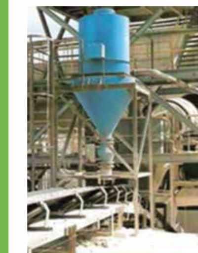
Intercept cyclonic hopper discharging on conveyor for re-cycle.
