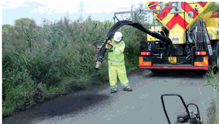
The aggregate mix is fired at high velocity through a delivery hose, evenly coating the aggregate granules with bitumen emulsion.
