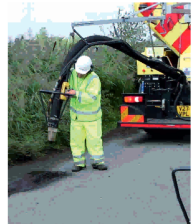
A cold bitumen emulsion is forced into every cracks and crevice, sealing the defect and protecting it by preventing the ingress of water.
